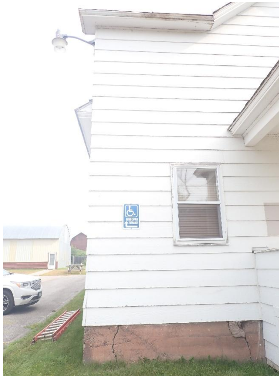
Photo 1: Vertical Cracks at SW Building Foundation
