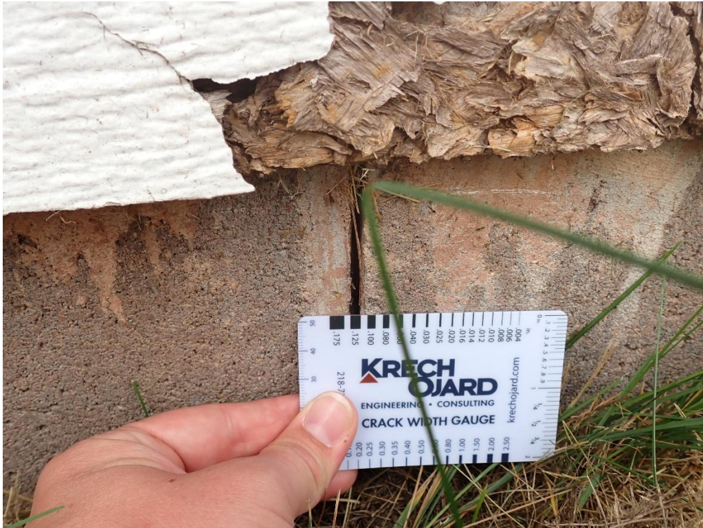
Photo 33: Addition – Separation at CMU Vertical Grout Joint at East Wall
