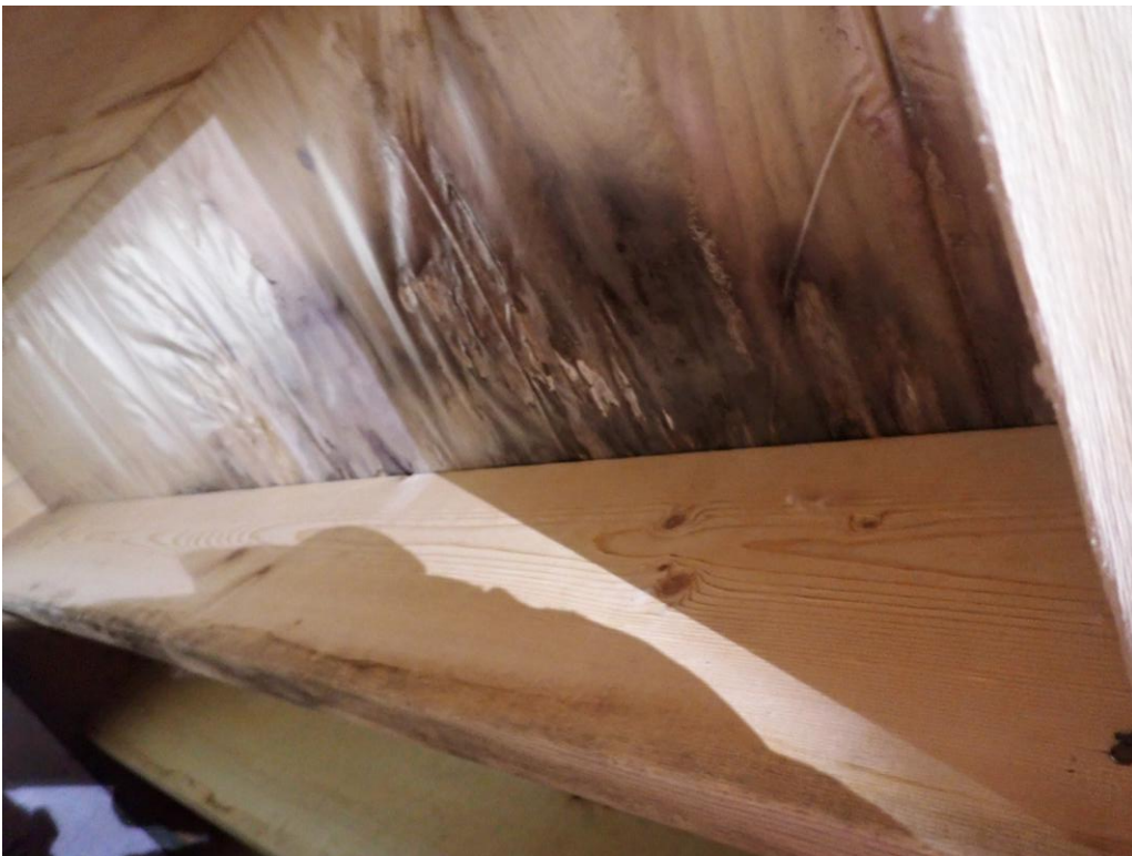
Photo 42: Addition – Moisture Staining in Floor Decking
