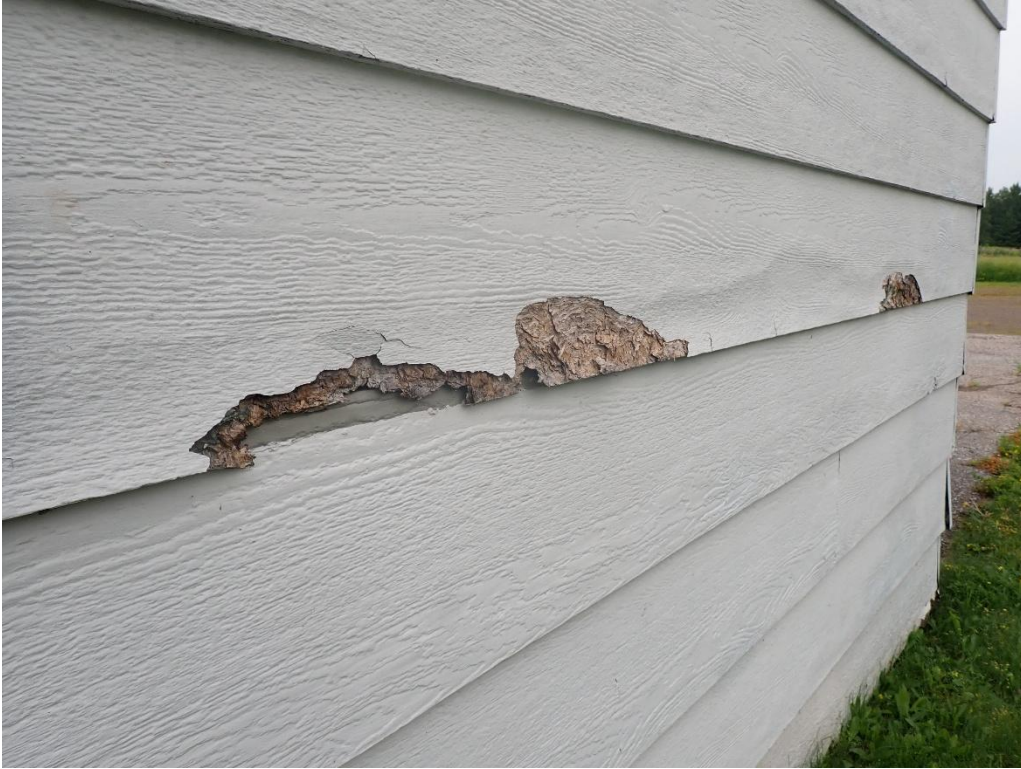
Photo 47: Example of Deteriorating Siding
