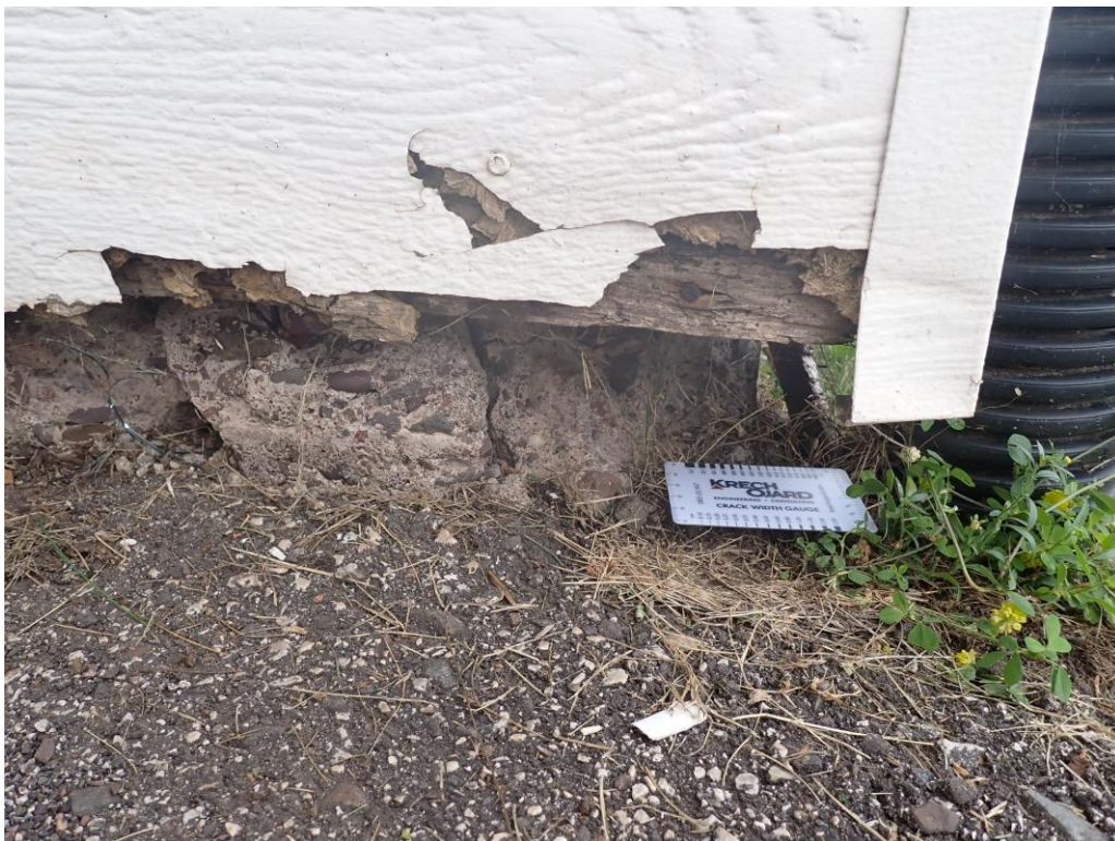
Photo 6: Spalling at NE Building Foundation Corner
