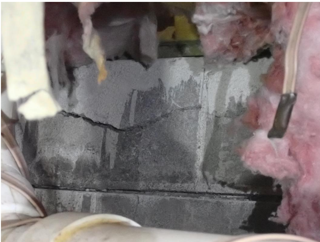
Photo 38: Addition – Horizontal Cracking through the CMU and at CMU Joint at the West Wall
