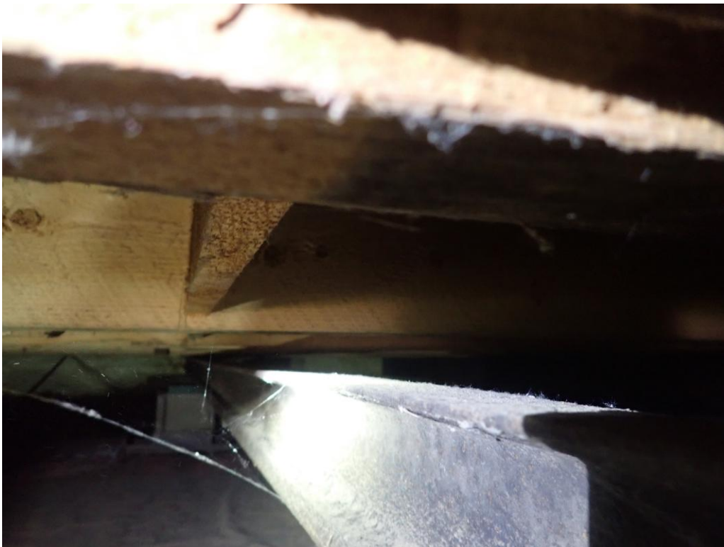
Photo 10: Pedestal Settlement – Gap between Rail Beam and Floor Framing (West)
