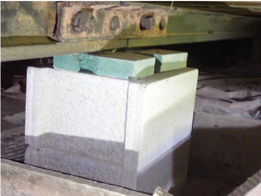
Photo 14: Pedestal Stone Cracking (P15)
