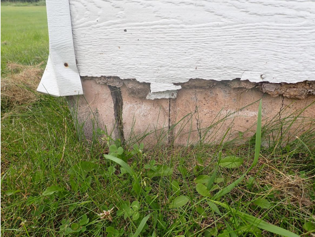
Photo 35: Addition – Cracking and Broken CMU Block at the NE Corner
