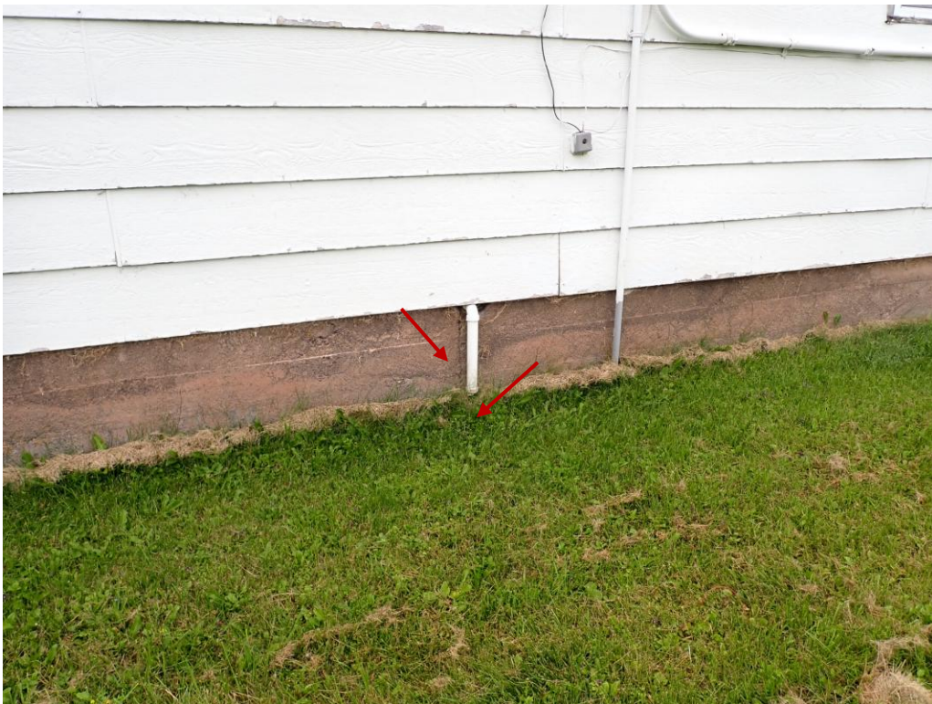
Photo 8: East Foundation Wall – Crack and Broken Pipe
