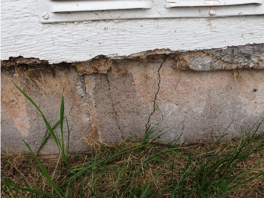
Photo 31: Addition - Cracking at CMU 2/3-3/4 Along the East CMU Wall
