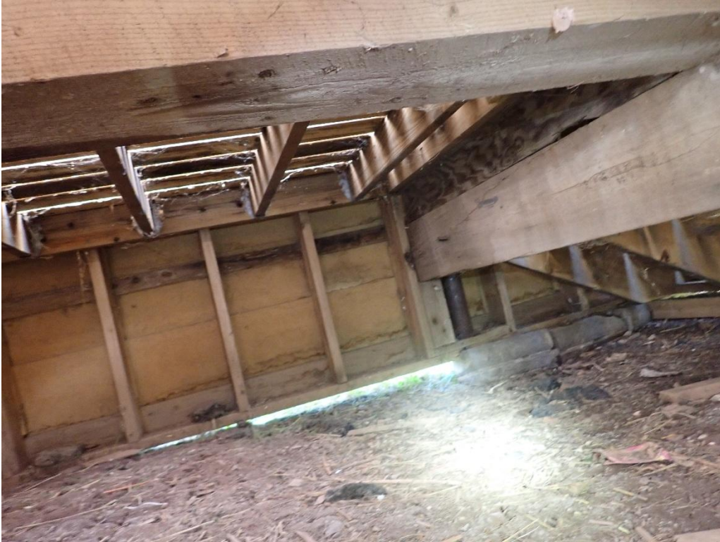
Photo 29: Damaged and Tipping East Porch Post Foundation
