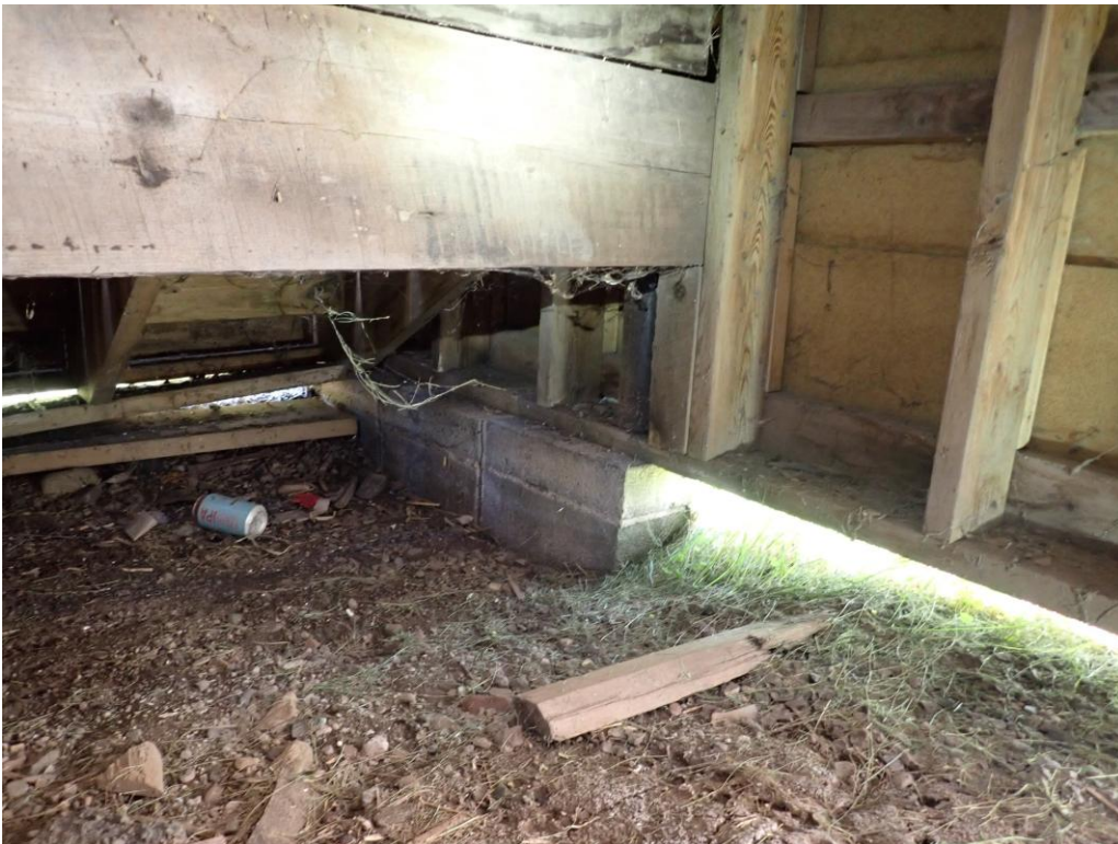
Photo 26: SW Porch Post CMU Foundation
