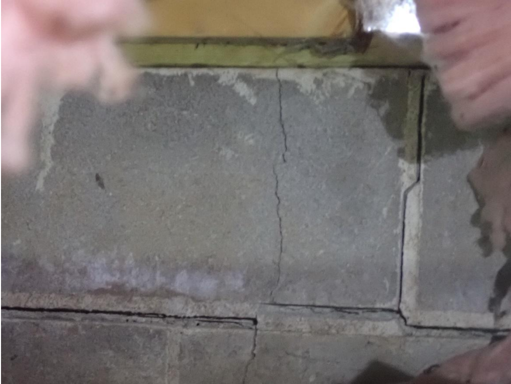
Photo 39: Addition – Vertical and Horizontal Cracking in CMU and Joints at the West Wall
