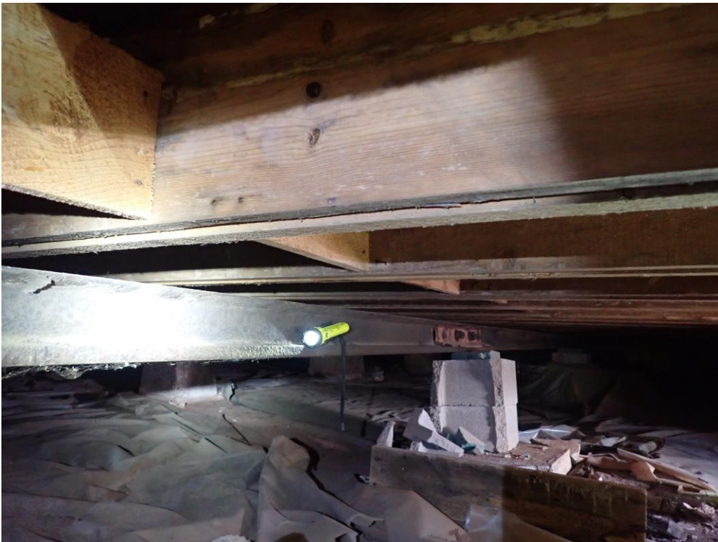
Photo 12: Pedestal Damage (P10)
