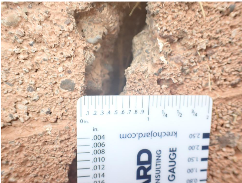
Photo 2: Crack at SW Building Foundation
