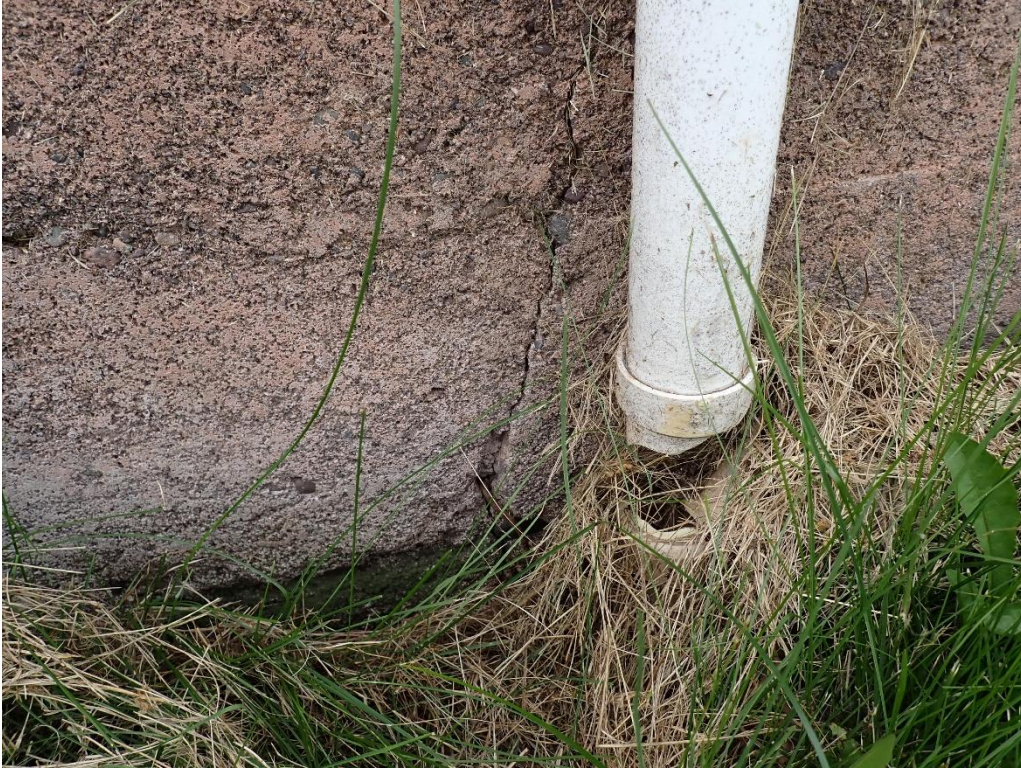
Photo 45: Broken Drain Pipe at East Wall (Outside of Kitchen)
