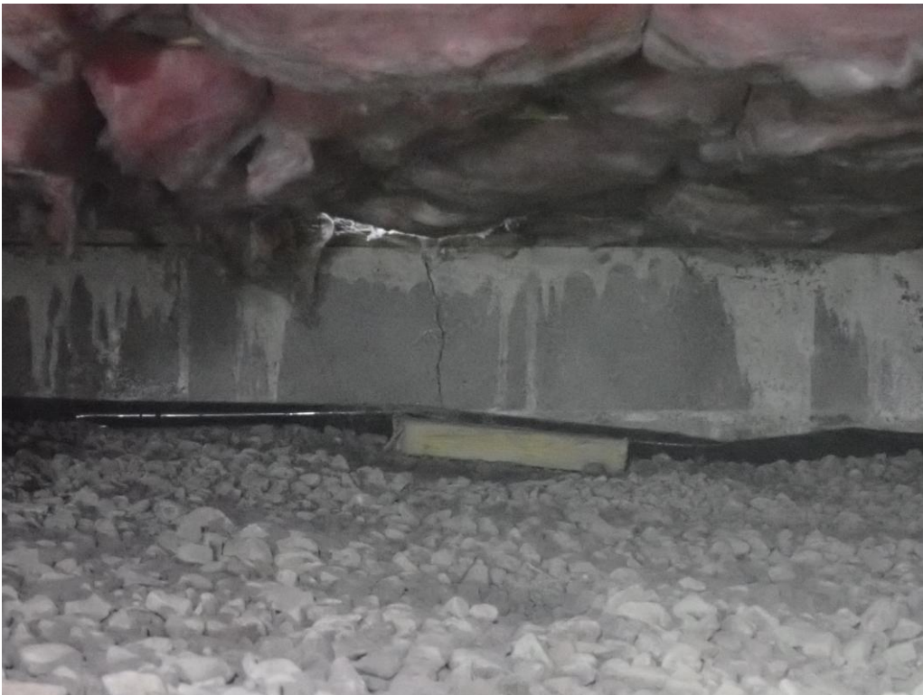
Photo 32: Addition - Cracking at CMU 2/3-3/4 Along the East CMU Wall
