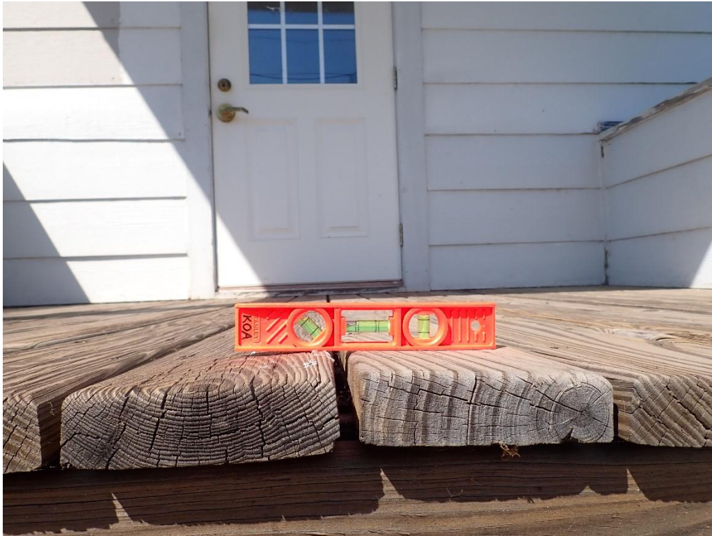
Photo 27: Porch Sloping Towards East
