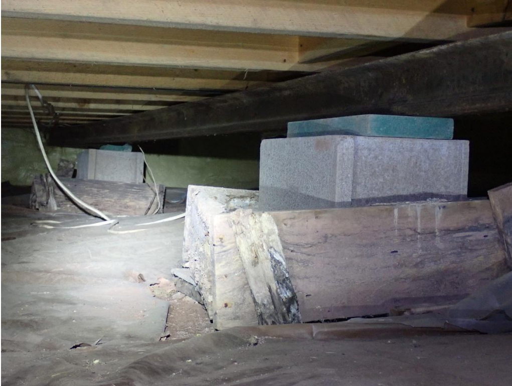
Photo 11: Pedestal Settlement – Gap between Rail Beam and Floor Framing (East)
