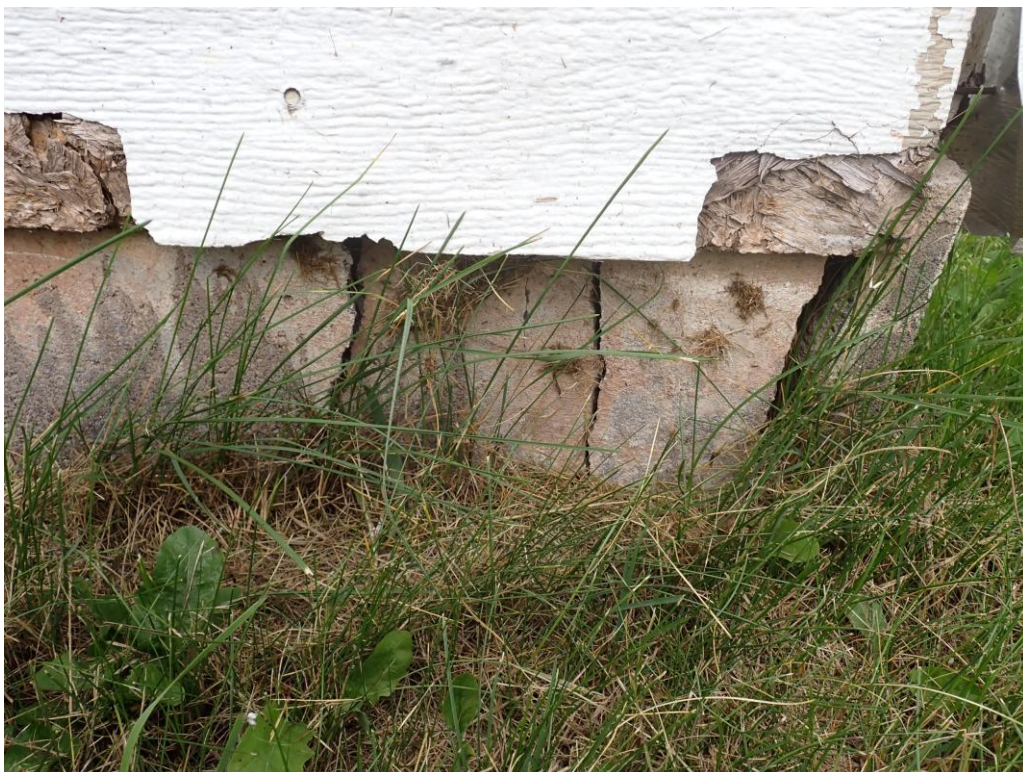
Photo 34: Addition – Cracking and Broken CMU Block at the NE Corner
