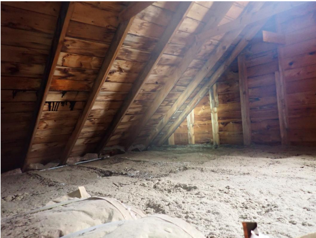
Photo 24: Moisture Staining at Roof – Original Building
