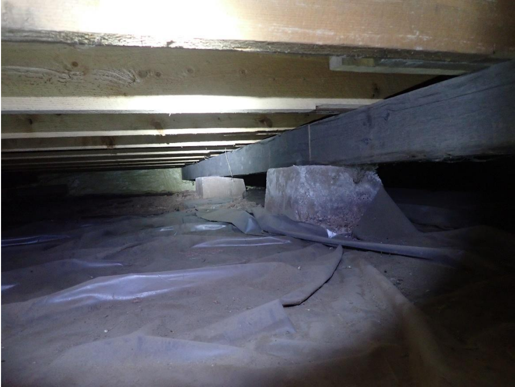
Photo 15: Spalls at Top of Pedestals P1 and P2
