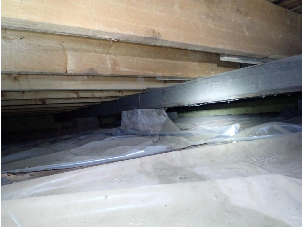
Photo 21: Checks in Timber Beam
