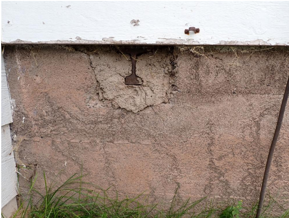
Photo 4: Crack at SE Building Foundation at Beam Bearing
