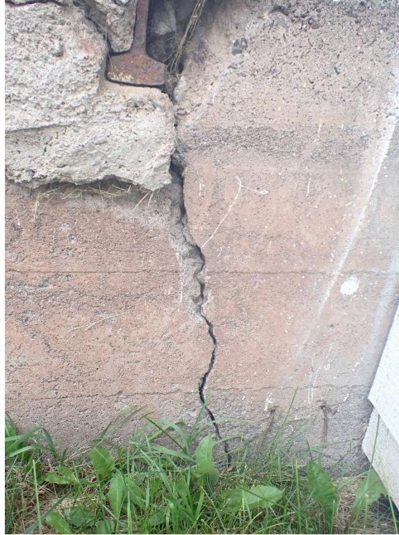
Photo 3: Vertical Cracks at SW Wall & Grout Spalling at Beam Bearing
