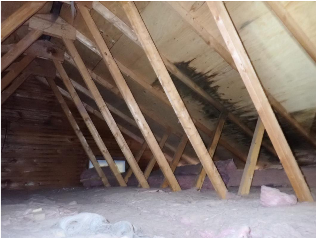
Photo 44: Addition – Attic Roof Moisture Staining at West Decking
