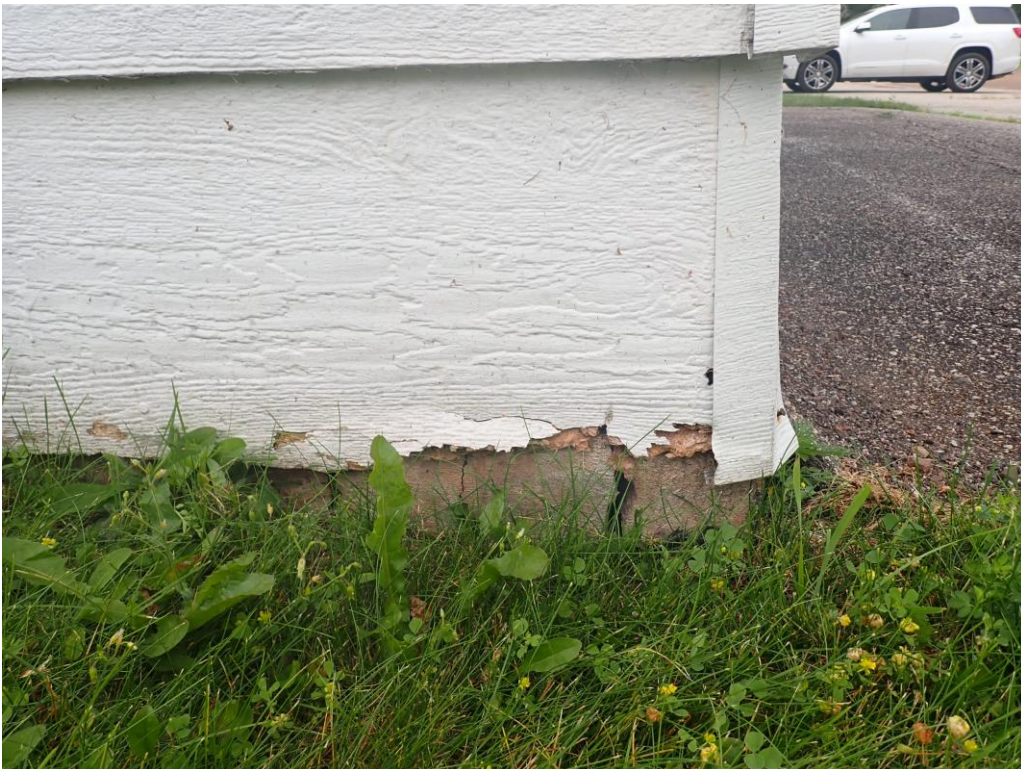
Photo 36: Addition – Cracking and Broken CMU Block at the NW Corner
