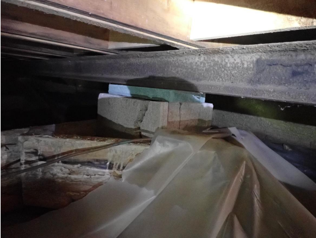
Photo 13: Pedestal Damage (P11)
