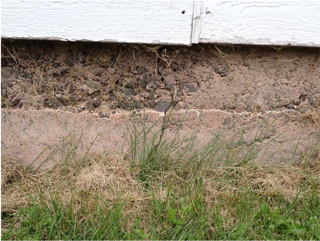
Photo 9: Crack at East Foundation Wall
