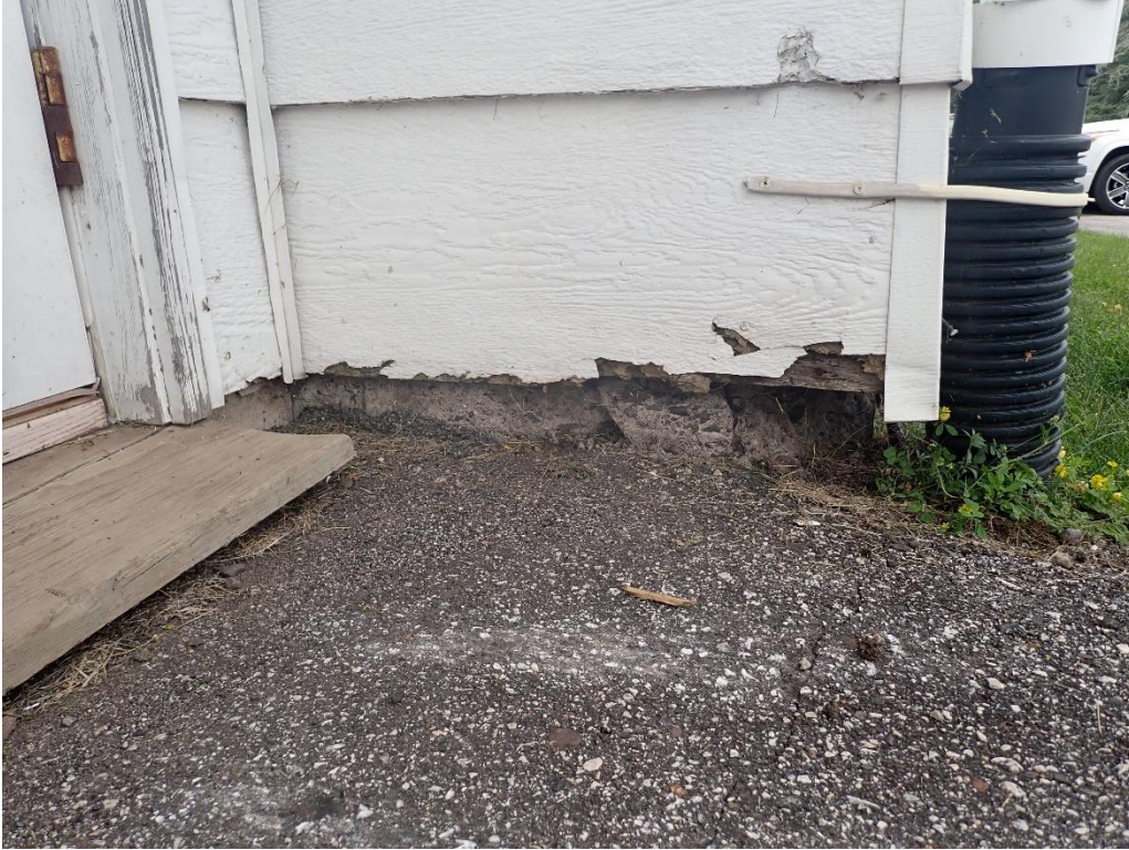
Photo 5: Spalling at NE Building Foundation Corner
