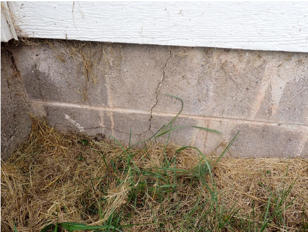
Photo 30: Addition – Cracking at the SE CMU
