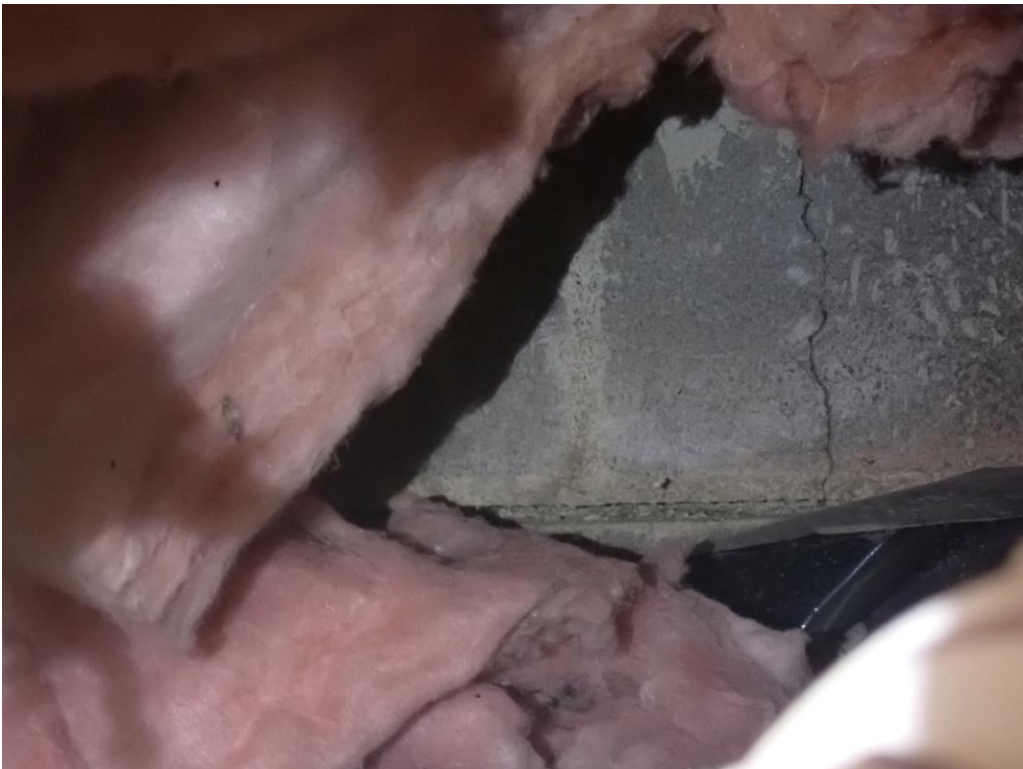
Photo 40: Addition – Vertical and Horizontal Cracking in CMU and Joints at the West Wall
